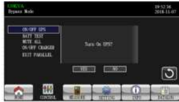
TURN OFF UPS
