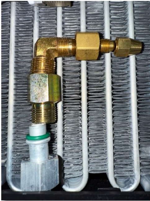
1/4" copper tube connects to filter/dryer/evaporator
