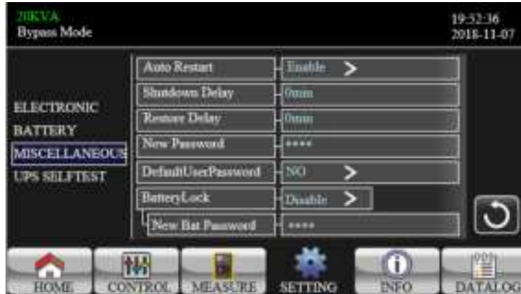
SCREEN: SETTING → ADVANCE → SERVICE → MISCELLANEOUS
